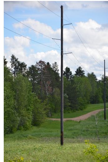
Typical 115 kV wood structure
